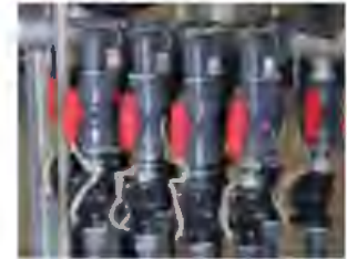
Manifold Housing and Water Hammer Arrester
